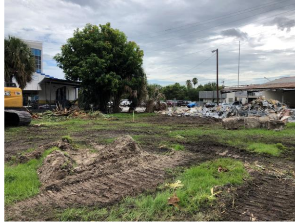
Where did all this debris come from!?
